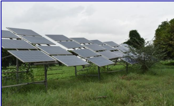
Solar Photo Voltaic Unit
