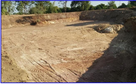
Rain Water Harvesting System
